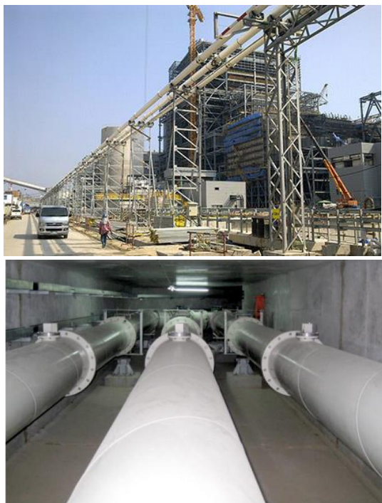
Figure 1 - GIL installations in power stations; above ground (left), and underground (right)
